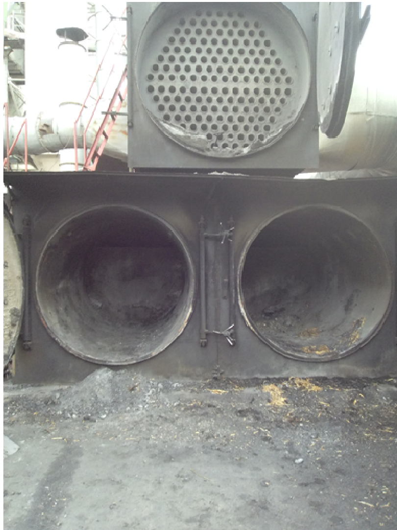
Fig. 1. General view of thermal generator for straw combustion
